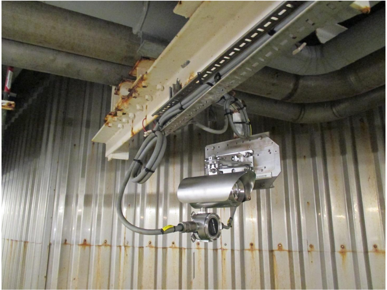
Figure 13. An ELDS™ transmitter unit installed on the main deck of the Terra Nova FPSO.
