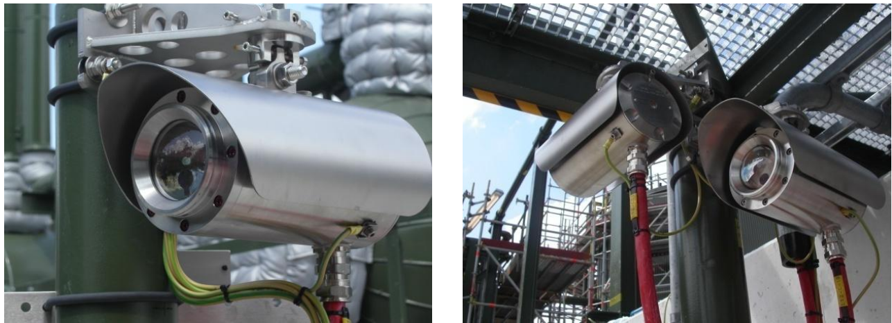
Figure 7. ELDS™ systems installed in field operations.
