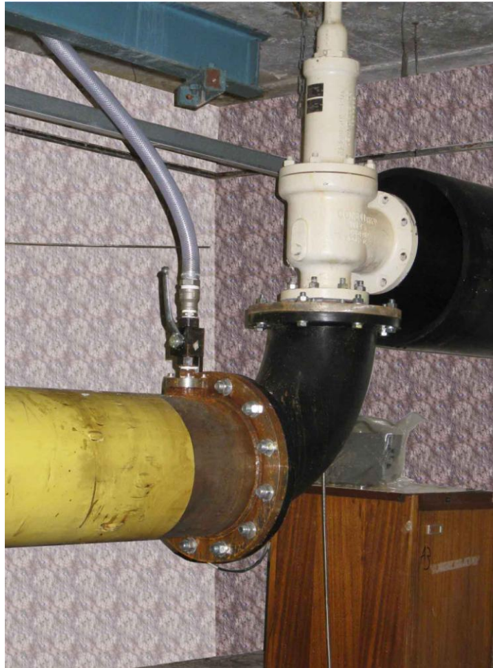
Figure 3. Relief valve (N) located at end of the water filled tube, also showing water outlet used for water filling and valve air bleed leg.
