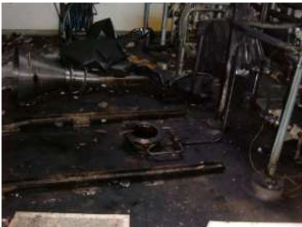
Figure 3: 3 rd floor charge chute
