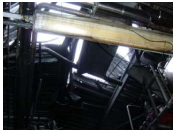
Figure 4: 3 rd floor roof damage
