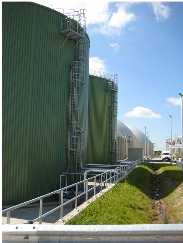
Figure 2. Barkip AD plant primary and secondary digesters
