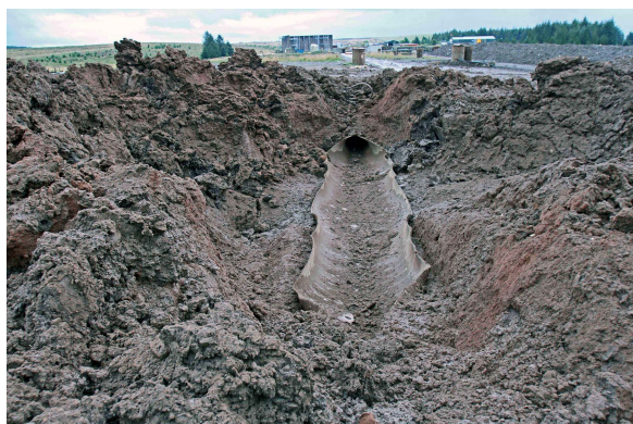
Figure 1. View of crater formed during instrumented burst tests on a buried section of pipeline
