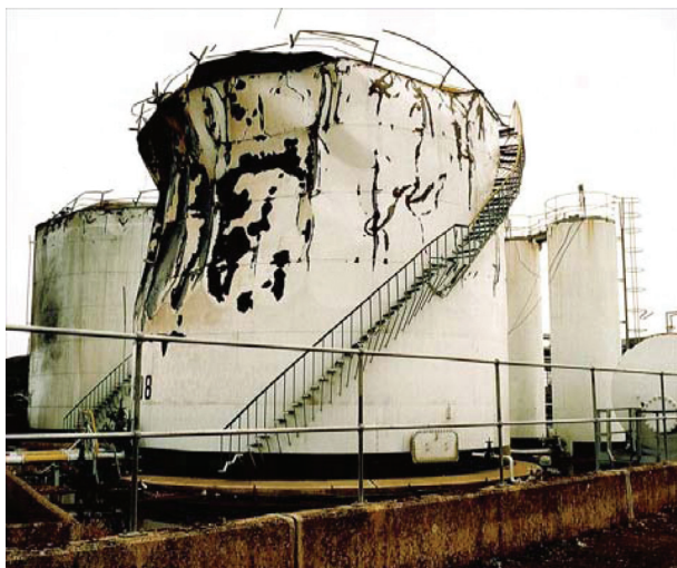
Figure 11. Front (North) face of Tank 908 showing extensive plastic deformation
