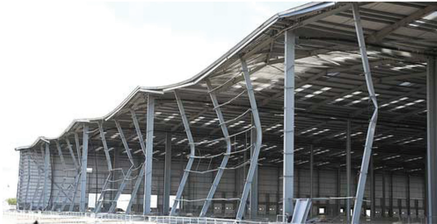
Figure 2. Warehouse 1 after remains of cladding removed
