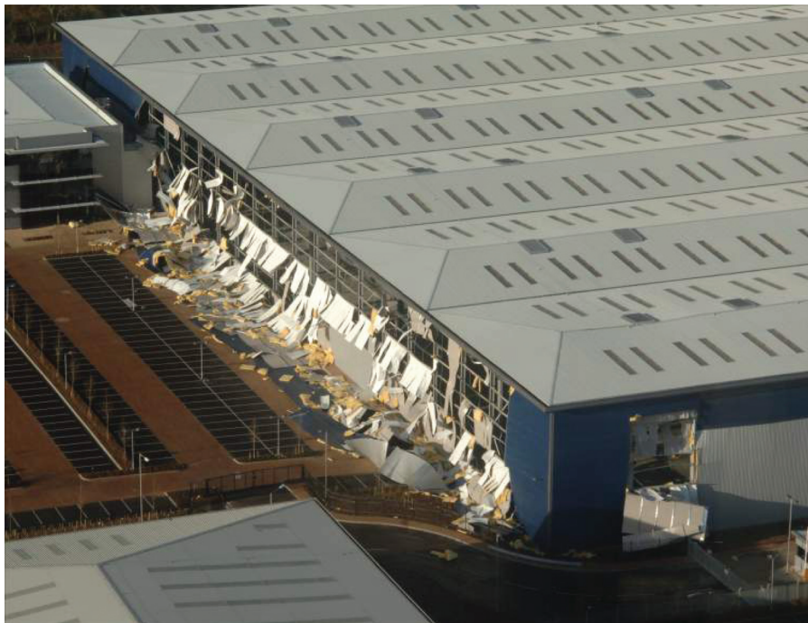
Figure 4. Warehouse 1 showing outward displacement of cladding on or near the back wall by an internal pressure surge
