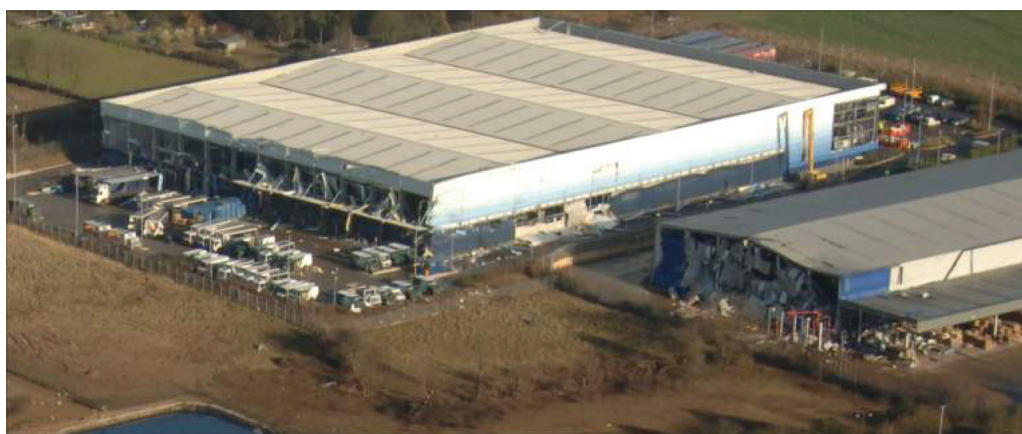
Figure 6. Warehouse 2 showing inward venting of front face and outward cladding loss on the back face caused by an internal pressure surge
