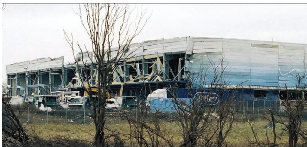
Figure 7. Warehouse 2 showing pressure damage to the (unvented) sidewall
