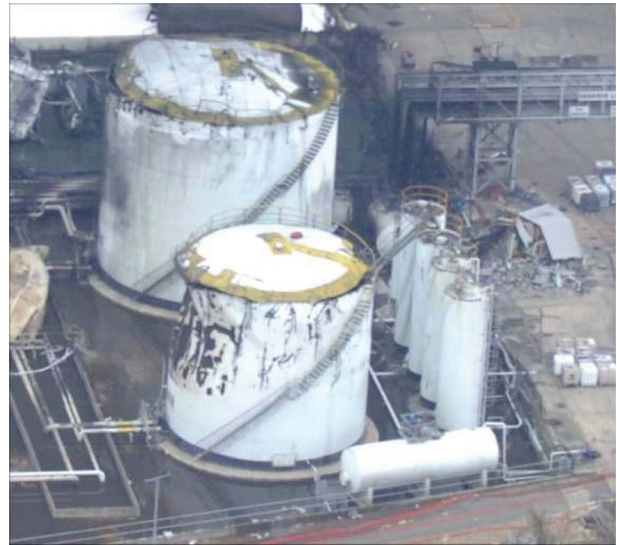
Figure 12. Side (West) face and roof of Tank 908. The weak, lightweight roof has bowed upwards at the end of the positive phase. E, W and S faces undeformed
