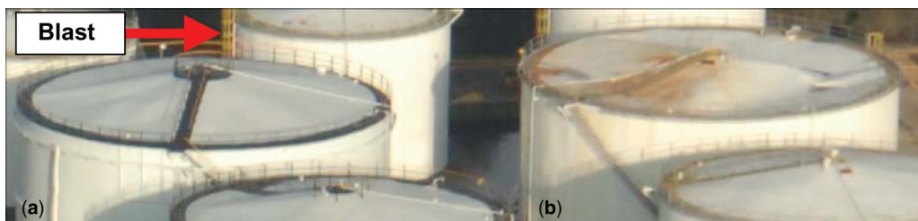
Figure 10. Deformation of tank tops outside the Buncefield cloud – Tanks A and B
