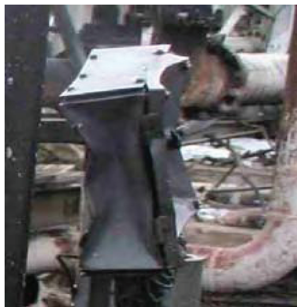
Figure 7. Crashed switch box at Buncefield (reproduced from Explosion Mechanism Advisory Group report, 2007)
