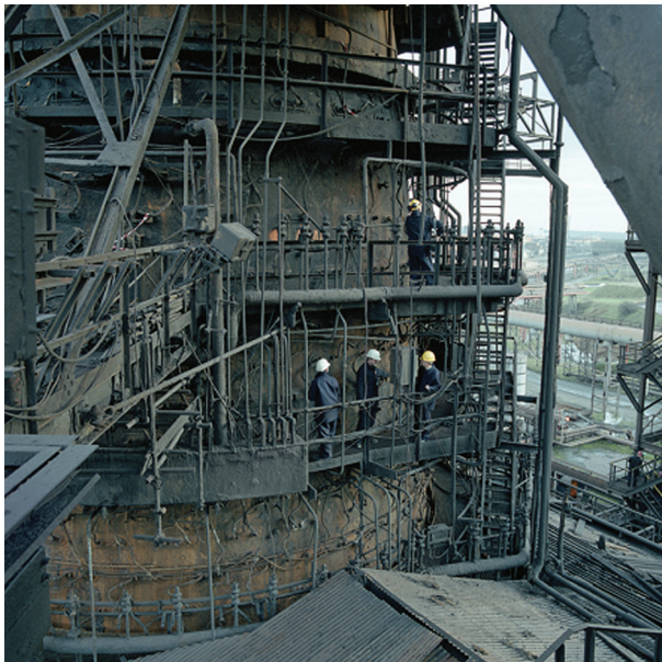
Figure 5. External view of furnace cooling system
