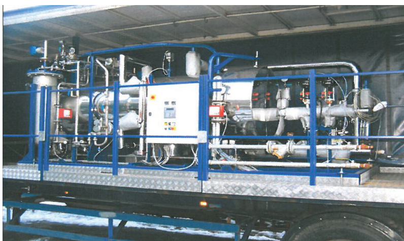
Figure 1. Typical thermal fluid installation (reproduced by permission of Heat Transfer Systems Ltd)
