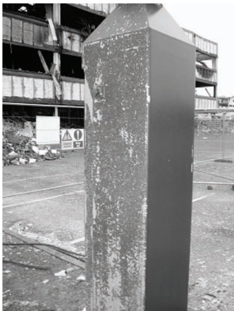
Figure 14. Directional abrasion of post
