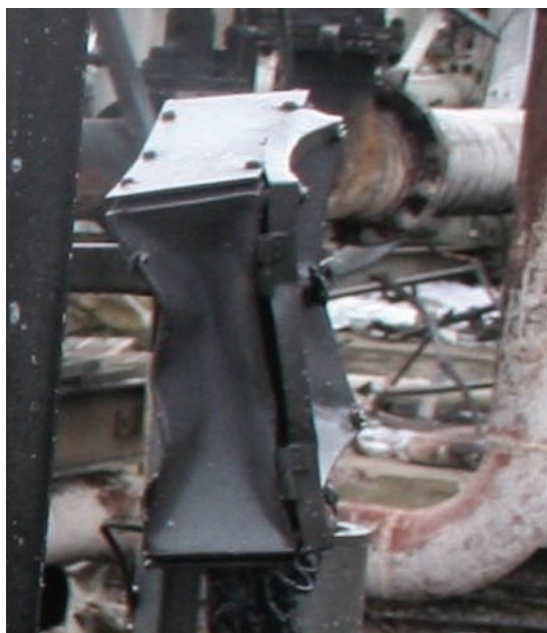
Figure 2. Junction box crushed by a severe VCE without demounting
