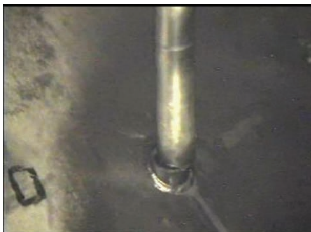
Figure 1. The fractured pipe on the accountancy tank
