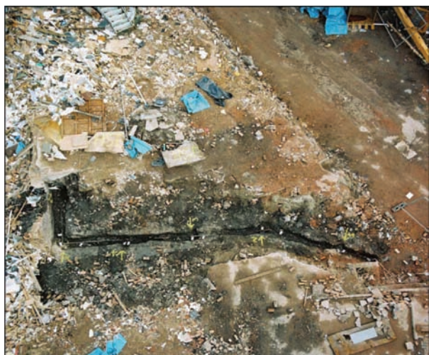
Figure 4. Excavated LPG pipe coming down from LPG torch (was bottom right but removed by this stage) to the basement wall visible centre left.
