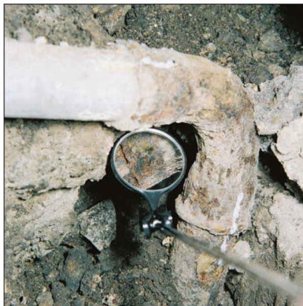
Figure 5. Photograph showing corrosion/crack in pipe elbow
