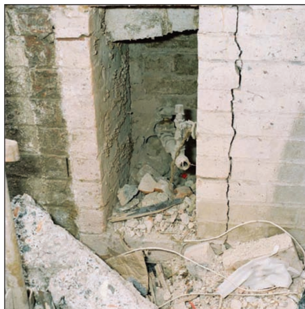
Figure 6. Shows the location of where the LPG pipe entered the basement. Note sheared off by building collapse
