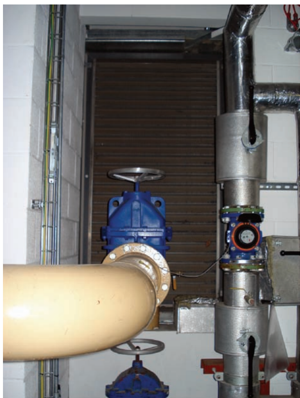
Figure 3. Gas inlet and ventilation louvre
