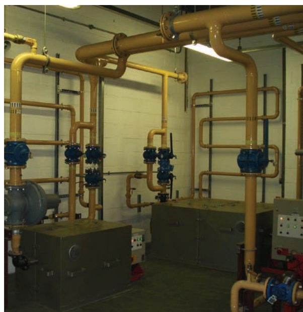
Figure 4. Manifolds and booster enclosures
