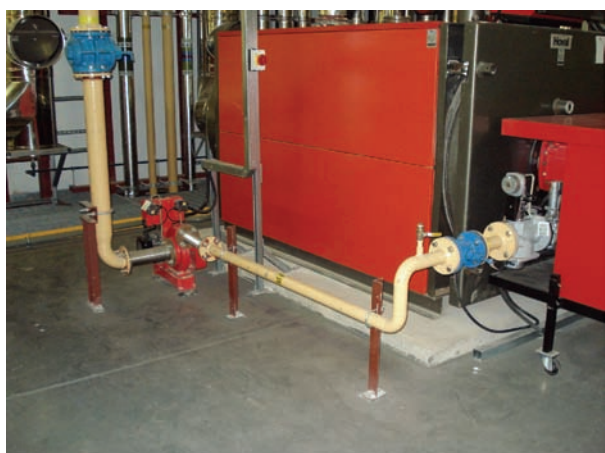
Figure 2. Boiler showing local booster
