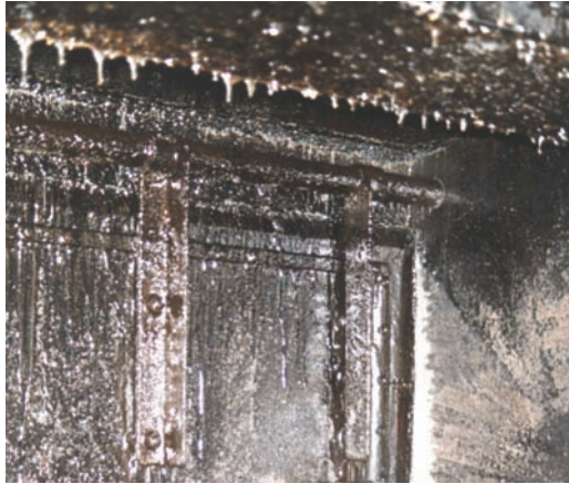
Figure 1. Appearance of tarry deposit in extract ductwork
