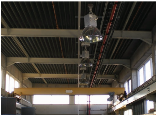
Picture 3. These light fittings descend from the ceiling so that the light bulb is easily replaced
