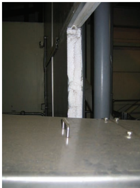
Figure 1. Expanded polystyrene insulation panel in thermal dryer building cut to allow conveyor access through side wall
