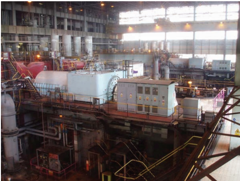
Figure 1. Typical turbine hall, showing two of the four generator sets
