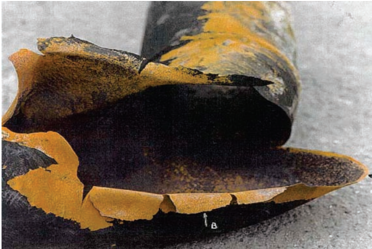
Figure 4. Photograph of the failed elbow showing the degree of pipe wall thinning
