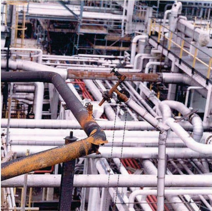
Figure 3. Photograph of the failed pipe elbow in situ showing the location of the water injection point
